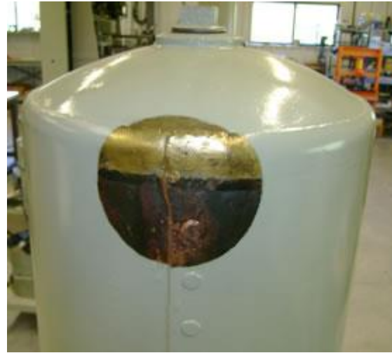
Figure 4. Brazed Tank – Outside
