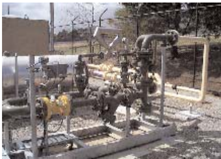
Figure 3. Master meter proving of a turbine meter using a 1" Coriolis meter.
