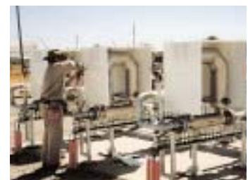
"After" installation since 1996, with two operating and one "hot spare" meter for 80:1 turndown. Custody transfer between utility and cogeneration project. 0.3 - 23 MMSCFD at 500 psia.
