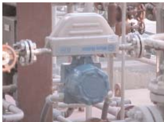
Installed R050 (1/2") meter
