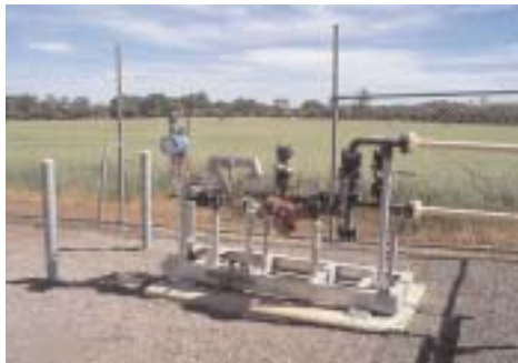
Distribution metering: 3.5MMscfd, 1000 psia, ModBus, high turndown.
