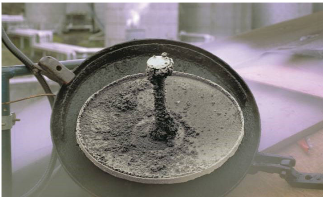
Figure 11: Antenna Exposed to Blown Bitumen for Several Months
