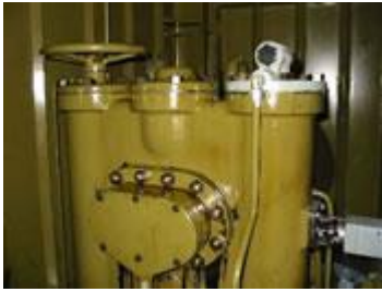
Figure 7. XX Pump Before
