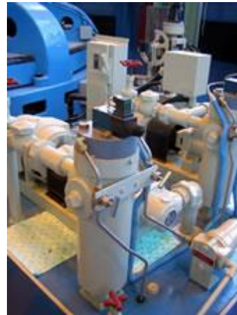
Figure 2. Replaced IMO Pilot Unloader Valve
