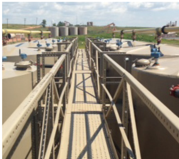
Rosemount 3308 Wireless Guided Wave Radars and Rosemount 2160 Wireless Vibrating Fork Level Switches installed on the water/oil tanks
