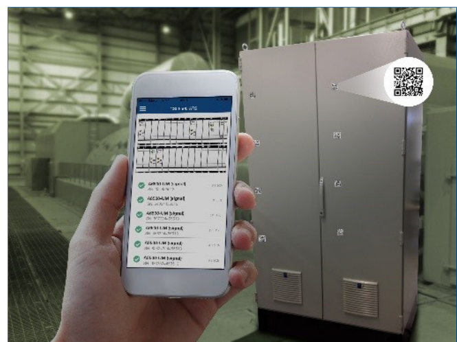
ATG View delivers asset health information to the user anywhere on the plant network.
