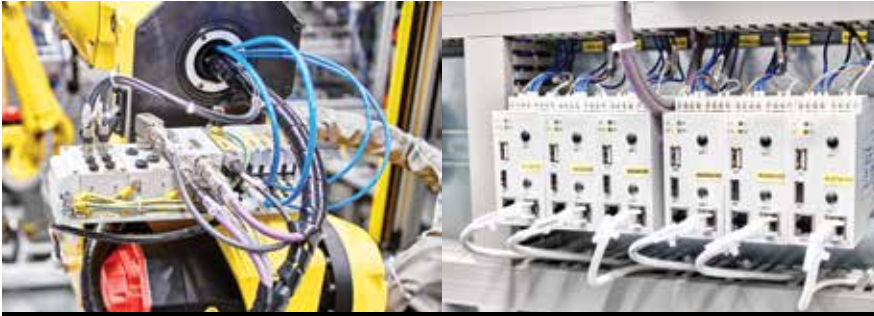
□ Valves with IIoT integration (left), connected to the smart pneumatic monitoring “hubs” (right) aggregate and organize pneumatic performance data and deliver it through separate, parallel pathways to plant management systems.
