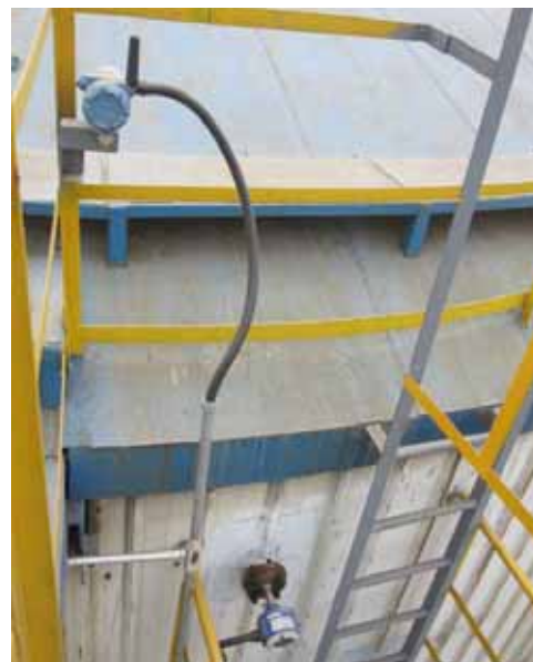
A Rosemount 702 Wireless Discrete Transmitter installed on top of a bitumen tank provides overspill protection.
