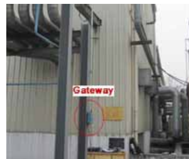
A Smart Wireless Gateway manages the wireless network.
