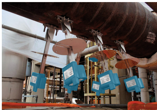
Figure 3. Real-time corrosion monitoring sensors in action.
