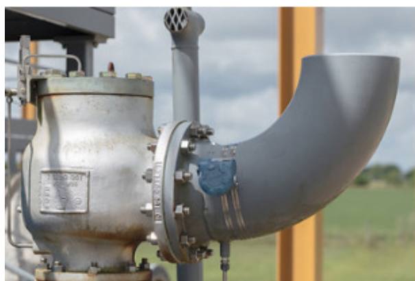
Figure 4. PRV online monitoring.
