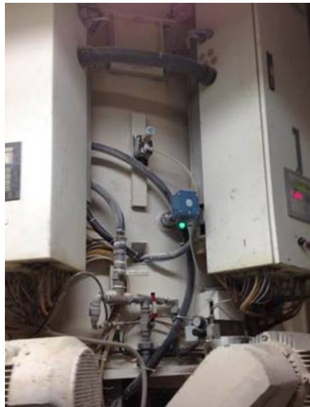
The Rosemount 2555 Solids Level Switch is installed in the Rotopack
