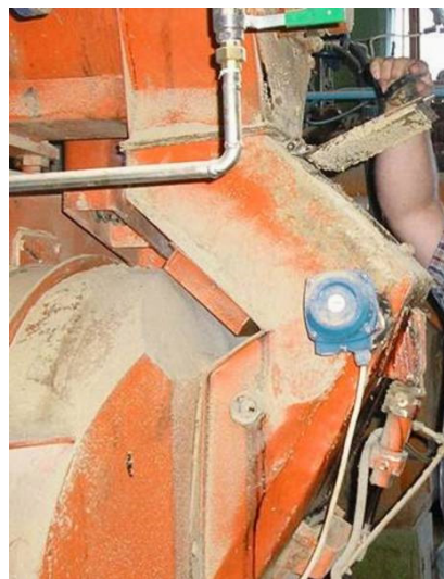
Rosemount 2511 installed on the animal feed hopper. Conditions are very dusty
