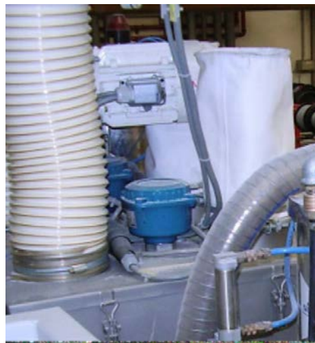
Rosemount 2501 is installed on the pre-holding vessel
