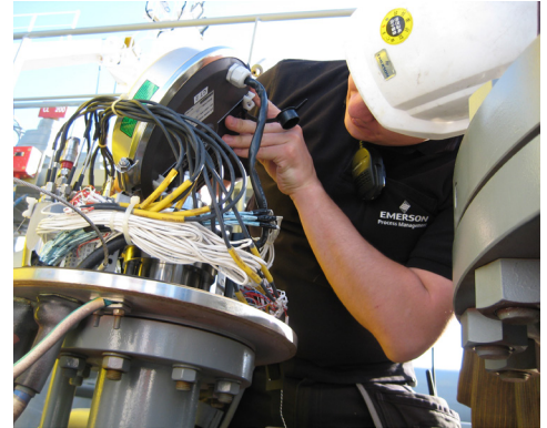
Overhaul is always completed by Emerson authorized service engineers.
