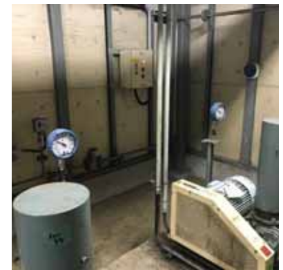
After the installation of Rosemount Wireless Pressure Gauges, the discharge pressure is continuously monitored at the operator station.
