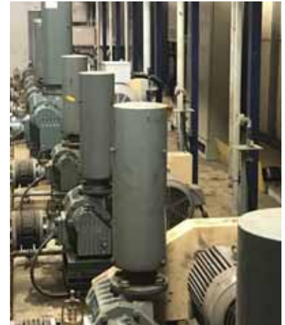
Before, with the existing mechanical pressure gauges, it was difficult, and potentially dangerous, to detect blower malfunctions.
