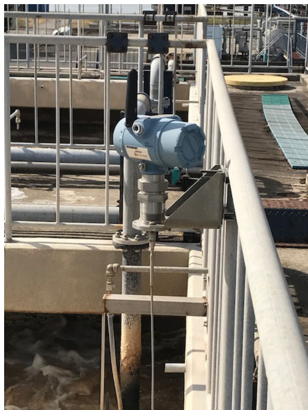
Rosemount 3308 Wireless Guided Wave Radar installed over the concrete pit.
