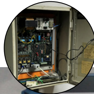
Before: With Legacy communication unit
