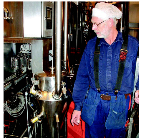
Image 1. Rosemount 2110 hygienic level switches mounted in the overspill tank.
