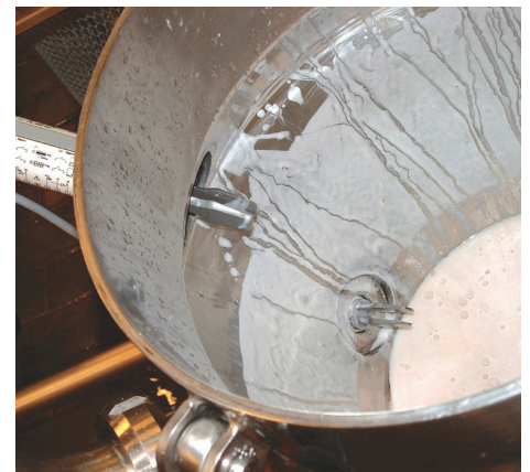
Image 2. Rosemount 2110 hygienic level switches mounted in the overflow tank.
