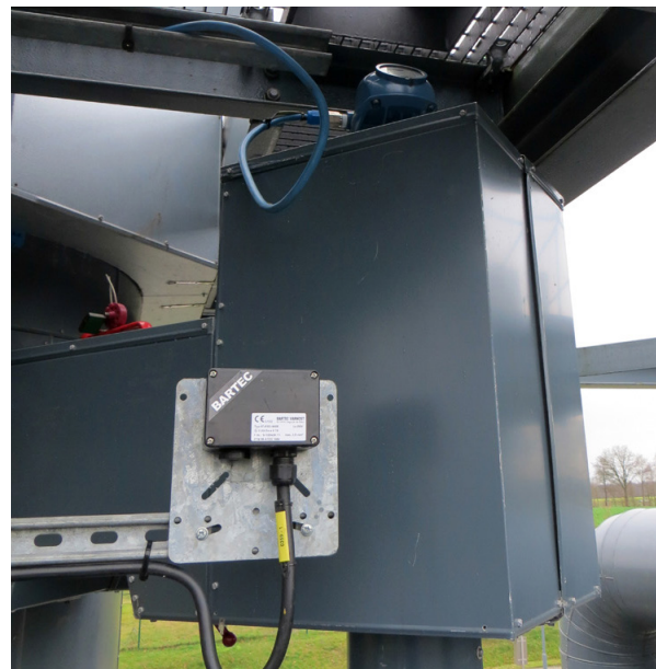
The Rosemount 5300 was installed in a chamber inside an insulated box.
