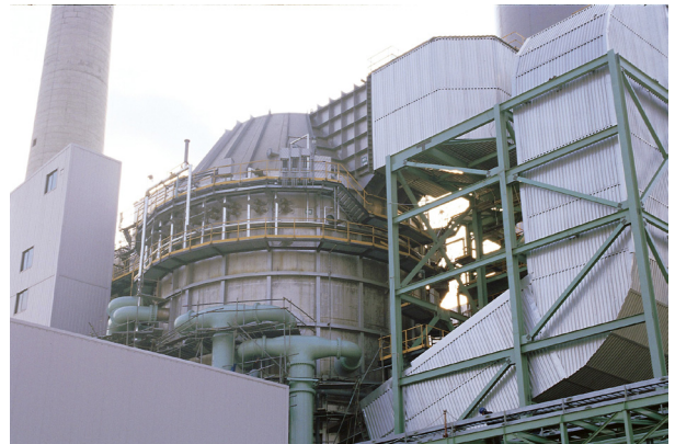
Use of technologies like a flue gas desulphurization system helps to secure Yonghung's place as one of the most clean and efficient power plants in the world.
