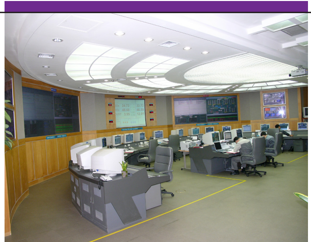
The main control room at the Yonghung Power Plant allows operators to view information pertaining to any process in the plant.
