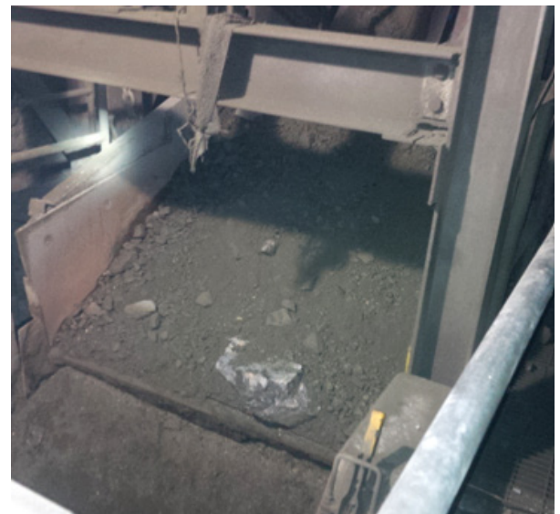
Dusty underground conditions
