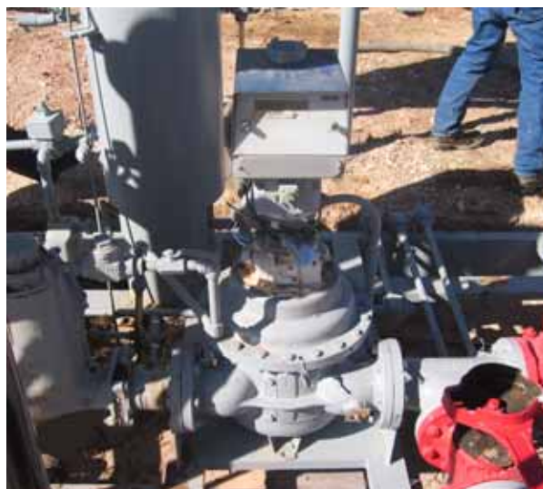
LACT system with a PD meter and external temperature compensator installed
