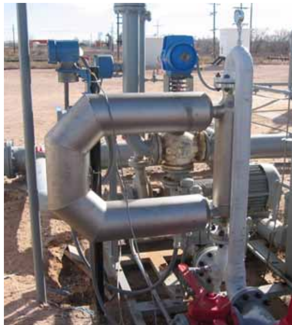
LACT system with a Micro Motion Coriolis meter (including a retrofit kit) installed as a direct replacement to the PD meter and temperature compensator
