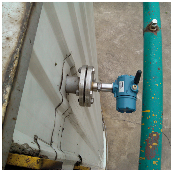
Rosemount 2160 Wireless Vibrating Fork Level Switch is mounted on the side of the fixed roof storage tank
