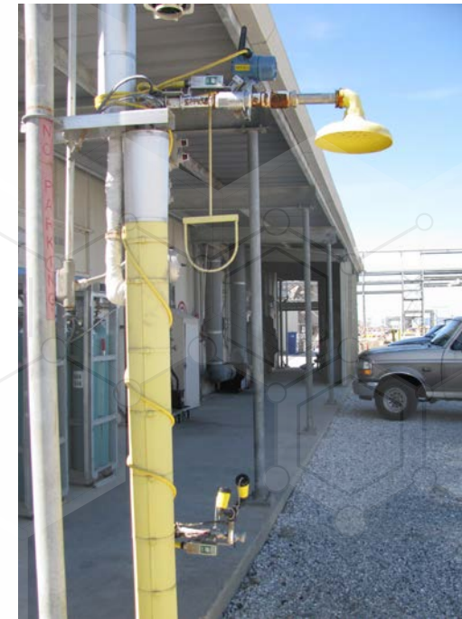
Figure 10: Adding a Rosemount 702 Wireless Discrete Transmitter can tell the control room which safety shower or eyewash station has been activated.
