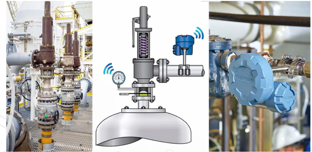
Figure 14: Rosemount 708 Wireless Acoustic Transmitters mount on piping adjacent to PRVs and steam traps to detect if they are functioning correctly or might be leaking. They are self-powered and send data via WirelessHART, so there is no need for any wiring.
