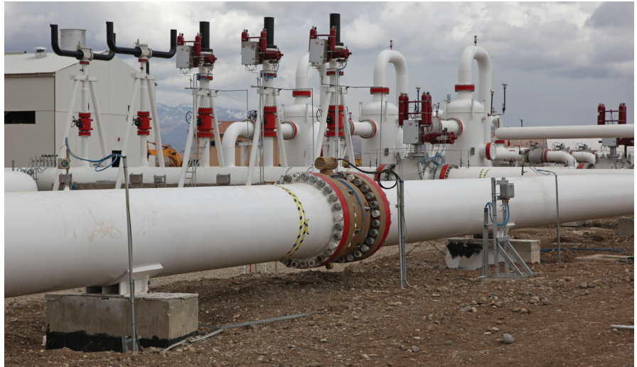
Figure 2. BOTAS natural gas compressor station at Çayirli, a town in the Erzincan Province of Eastern Turkey.
