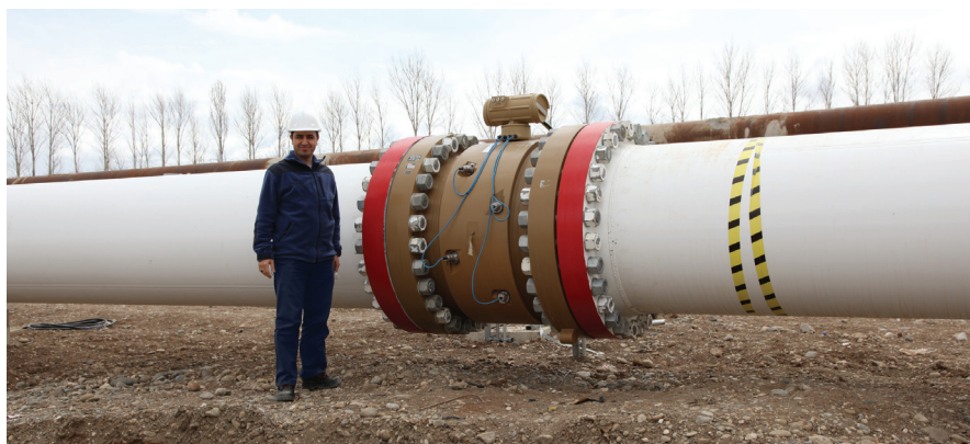
Figure 1. Daniel Measurement and Control's 42-inch SeniorSonic ultrasonic flowmeter installed in the BOTAS pipeline.
