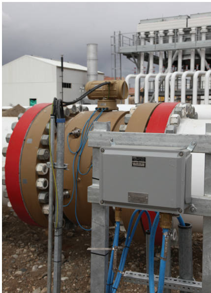
Figure 5. The availability of an accurate allocation metering system was a key requirement in the development of the new gas compression station that will serve the natural gas pipeline running across northern Turkey.
