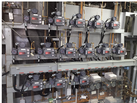
Figure 1: Liquid zone control valves at Pickering
