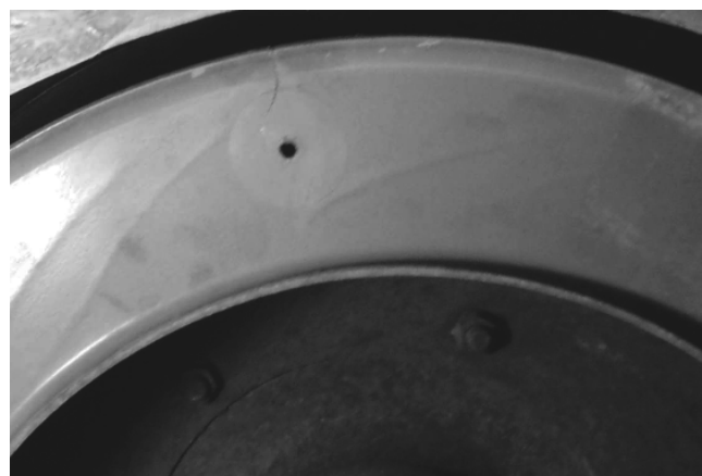
Fig. 8: Examination revealed a defect in the blower wheel.
