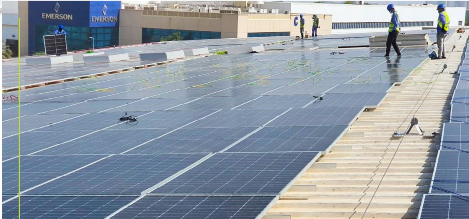
Emerson Dubai campus recently installed an on-site solar system that provides over half of its daily electricity usage.
